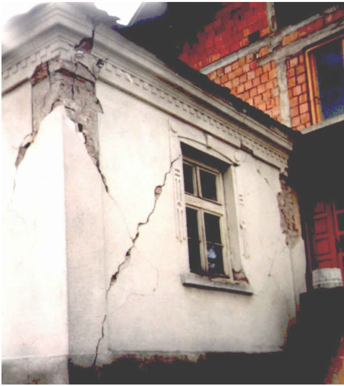
Damage to masonry buildings in the 1998 Mionica earthquake
