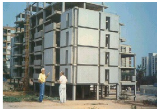
A building under construction, showing columns at the top floor erected in the vertical position
