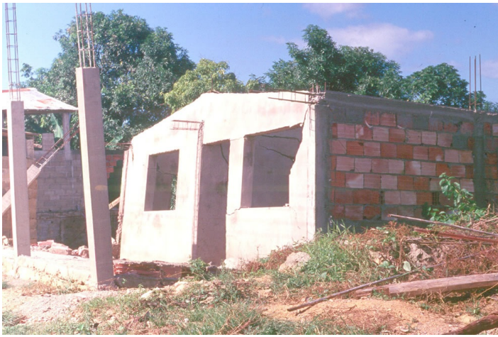
A Photograph Illustrating Typical Damage (1997 Cariaco earthquake)
