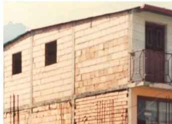
Inexistent Collar Beam
