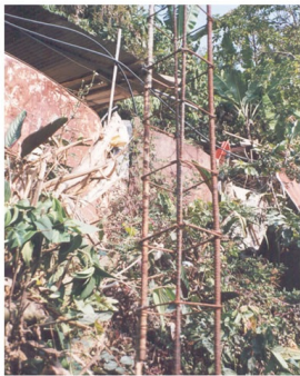
Ties and Stirrups widely spaced, 90 ° Anchorage hooks
