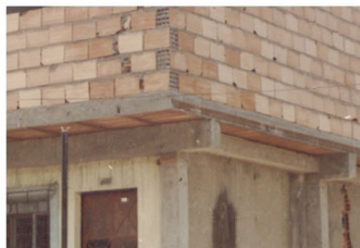
Inadequate connection between floor and frames
