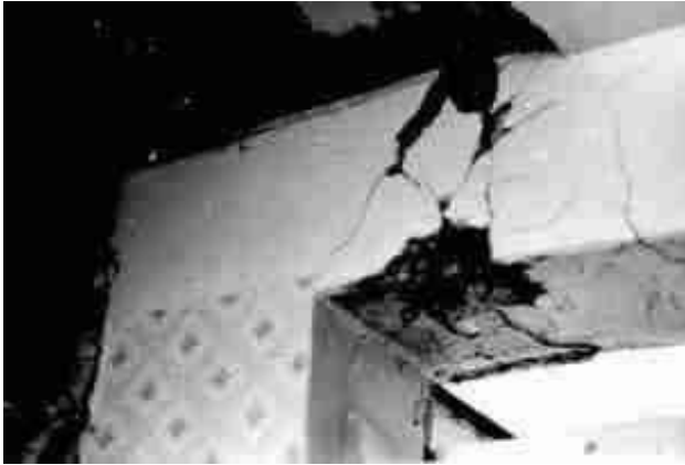
Building Damage in Leninakan (1988 Spitak, Armenia Earthquake)
