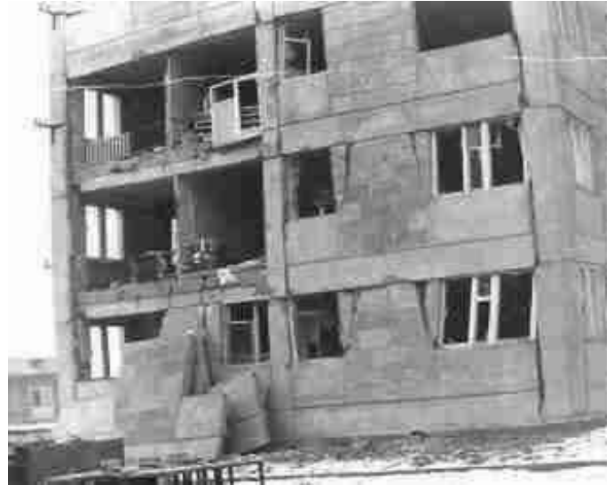
Building Damage in Leninakan (1988 Spitak, Armenia Earthquake)
