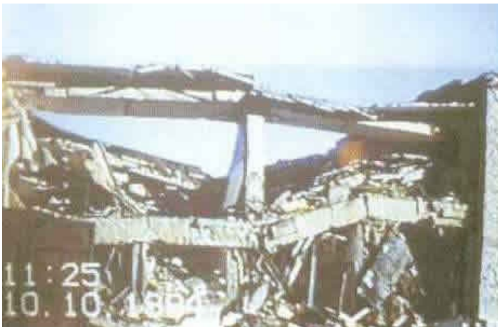
Building Damage (1994 Shikotansk, Russia Earthquake) Source: Klyachko 1999
