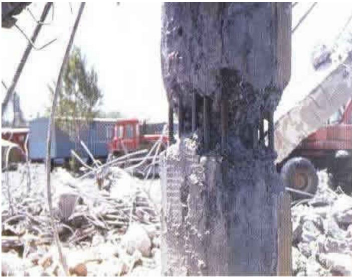
Building Damage (1988 Spitak, Armenia Earthquake)
