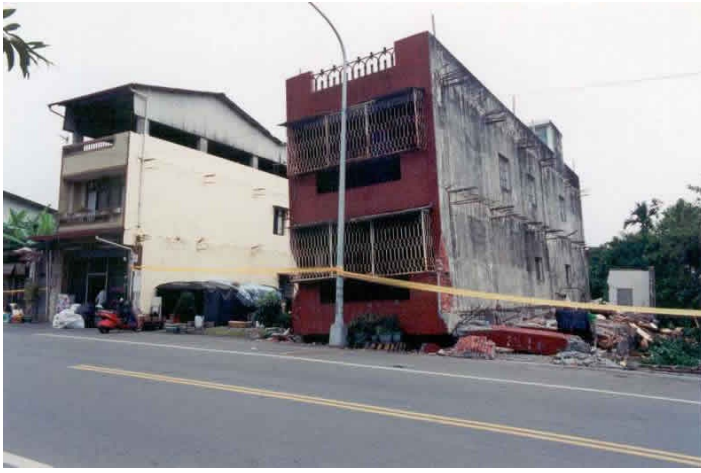
Earthquake damage - Collapsed Three-story building in the 1999 Chi Chi earthquake (Source: EERI 2001)
