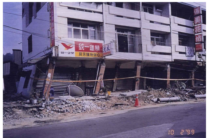
A Photograph Illustrating Typical Earthquake Damage
