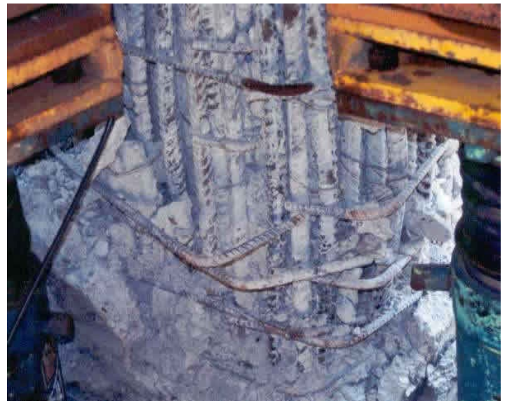
Earthquake Damage - Opening of 90 degree column hooks in the 1999 Chi Chi earthquake (Source: EERI 2001)
