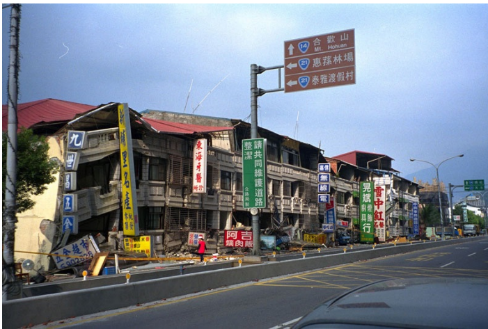
Earthquake Damage - Pancake Collapse of an Entire City Block in the 1999 Chi Chi earthquake (Source: EERI 2001)
