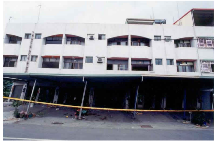
Earthquake Damage - Partial Collapse of a Three-story building in the 1999 Chi Chi Earthquake (Source: EERI 2001)
