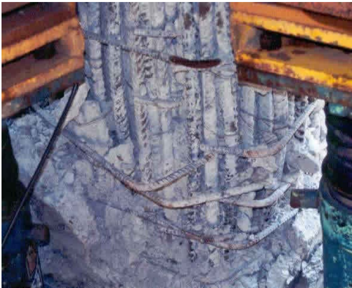
Earthquake Damage - Opening of 90 degree column hooks in the 1999 Chi Chi earthquake (Source: EERI 2001)
