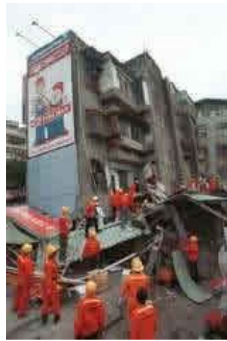
Earthquake Damage - Collapse of a 5-story building in the March 31, 2002 Taipei earthquake
