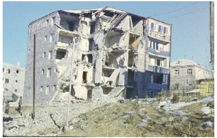
A Photograph Illustrating Typical Earthquake Damage (Spitak, Armenia earthquake 1988)
