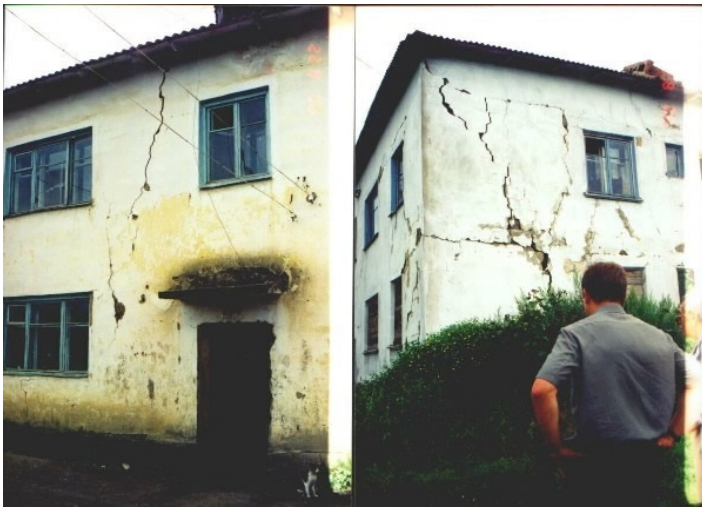
Typical Earthquake Damage
