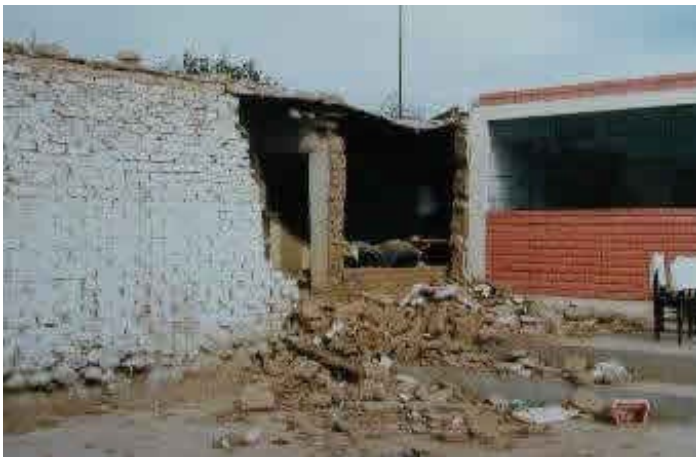
Key Seismic Deficiencies - Wall Damage Due to Inadequate In-Plane Seismic Resistance
