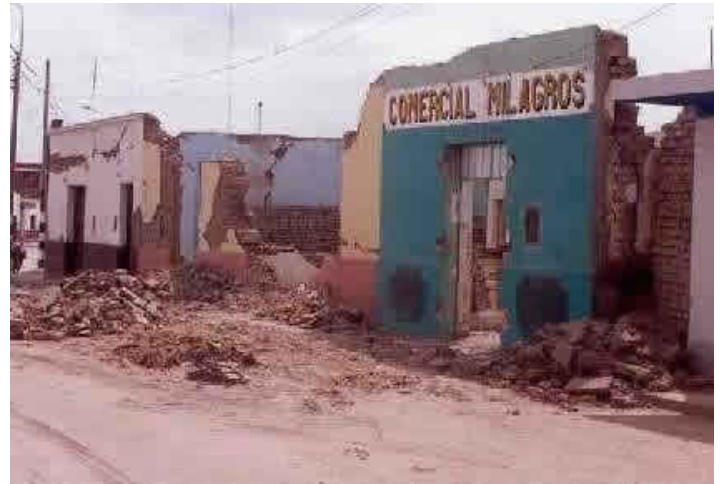
Key Seismic Deficiencies - Adobe Wall Failure Due to Out-of-Plane Seismic Forces
