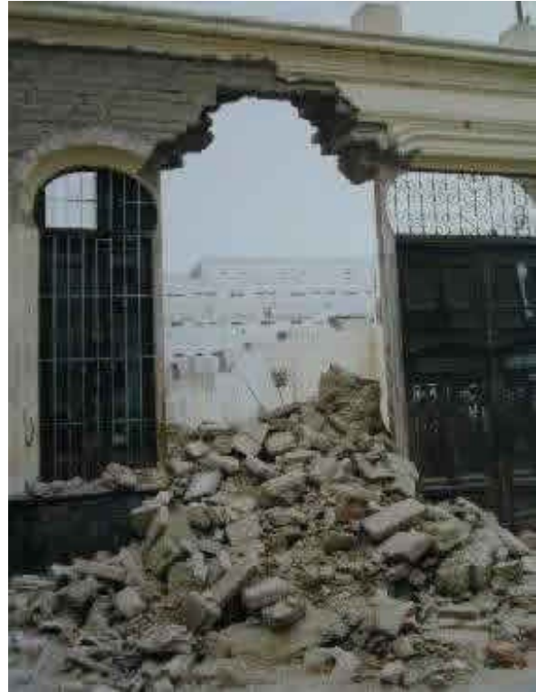
A Photograph Illustrating Typical Earthquake Damage (November 1996 Nasca Earthquake)
