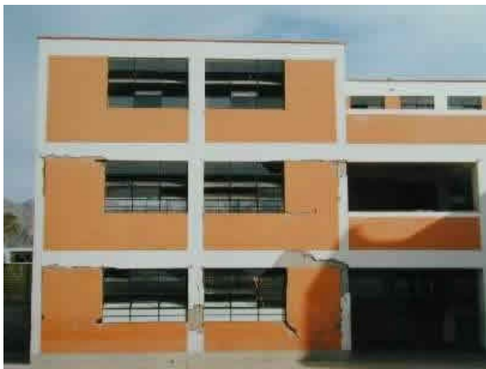
A Photograph Illustrating Typical Earthquake Damage (1996 Nazca earthquake)
