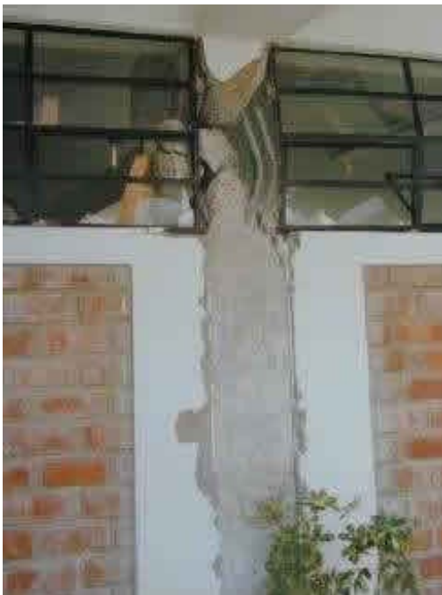
Seismic Deficiencies - Short Column
