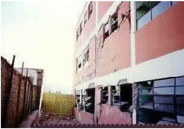
A Photograph Illustrating Typical Earthquake Damage
