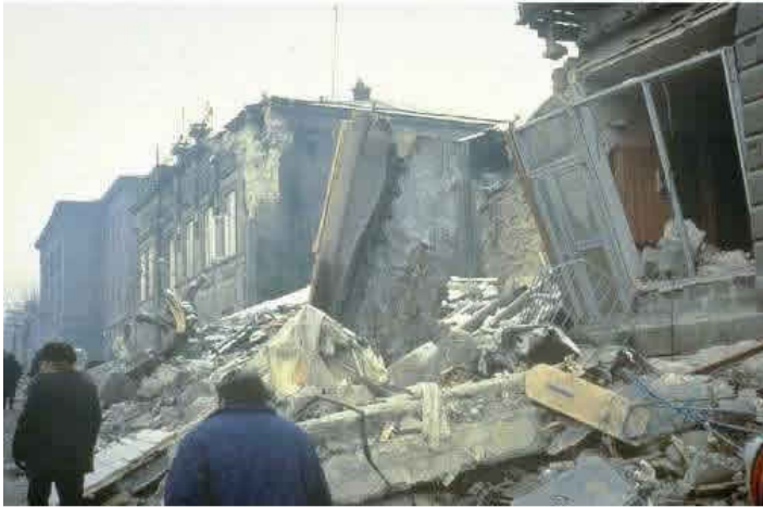
A Photograph Illustrating Typical Earthquake Damage (1988 Armenia earthquake, source: EERI Annotated slide collection)
