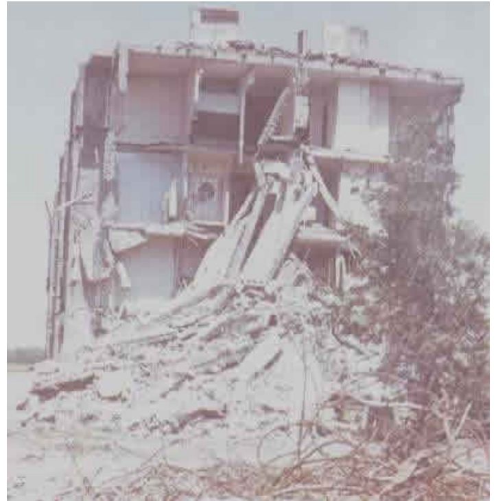
Building Collapse in the 1988 Spitak, Armenia Earthquake (Source: Klyachko, 1999)
