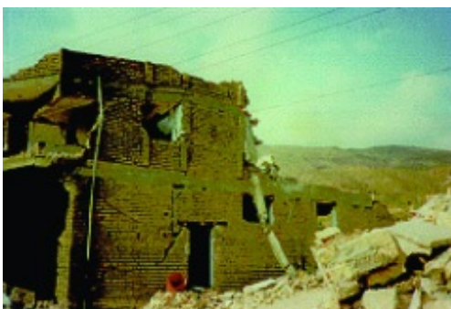
Damage caused by the absence of concrete posts (1990 Manjil earthquake)
