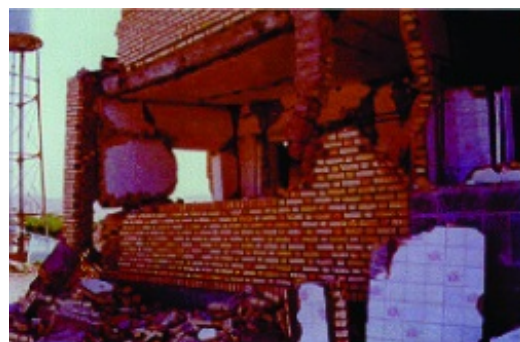
Damage due to large opening, absence of masonry shear wall and short column behavior in concrete post (1990 Manjil earthquake)
