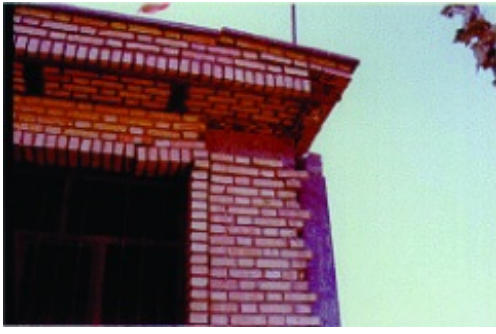
Damage in the wall panel (1990 Manjil earthquake)
