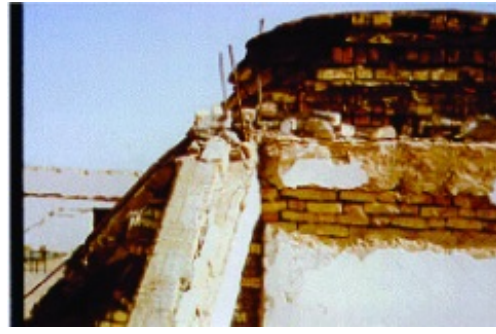
Collapse due to heavy roof (1990 Manjil earthquake)
