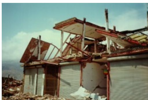
Building damage in the 1990 Manjil earthquake-collapse caused by the connection failure
