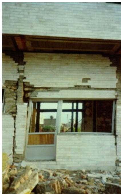
Failure due to soft story behavior in the 1990 Manjil earthquake
