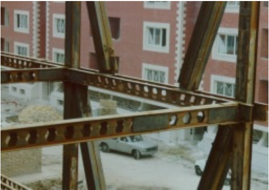
Seismic deficiency-use of undefined bracing system
