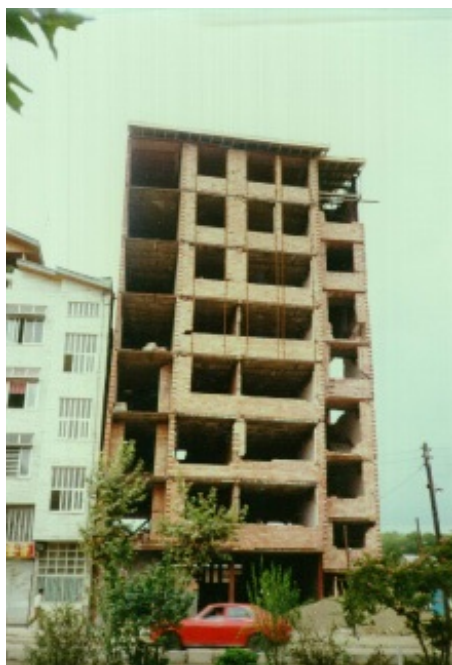
Minor damage due to pounding between two adjacent buildings in the 1990 Manjil earthquake
