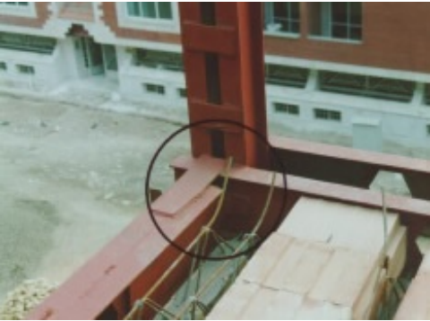
A seismic deficiency: wrong connection detail
