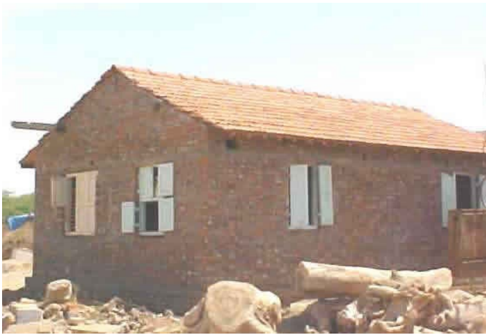
Key Seismic Resilient Features: RC Lintel Band and Good Quality Brick Masonry Construction (Source: Sudhir K. Jain, IIT Kanpur)
