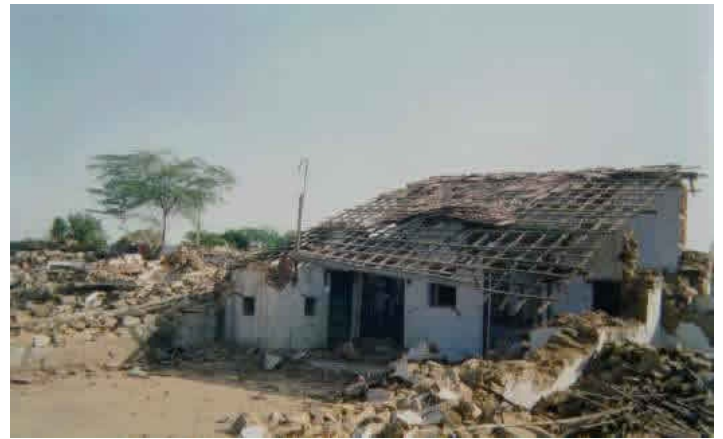
Failure of a Residential Building, Chobri Village near Bhachau, 2001 Bhuj Earthquake (Source: IIT Powai 2001)
