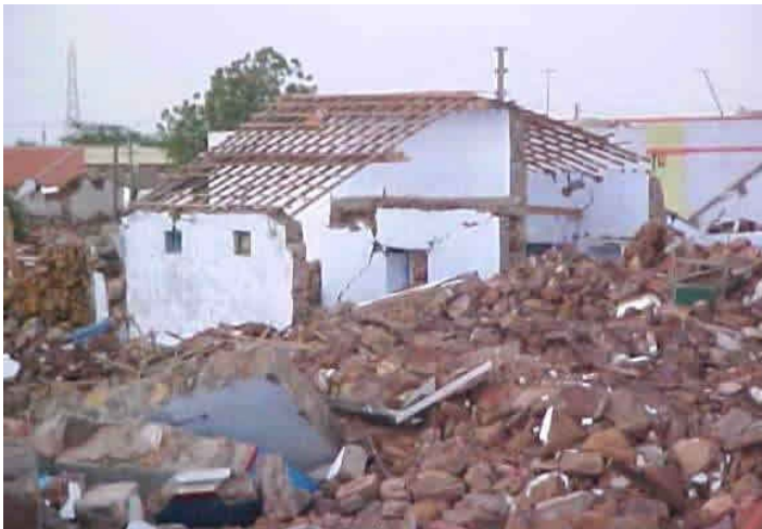
Typical Earthquake Damage: Collapse of Roof and Walls of a Brick Lime Mortar House in the 2001 Bhuj Earthquake (Source: Sudhir K. Jain, IIT Kanpur)
