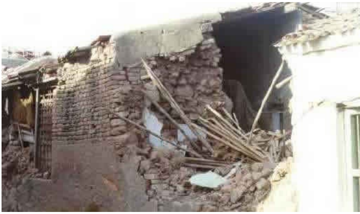
Typical Earthquake Damage - Wall Collapse Due to Poor Quality Brick Construction and Poor Inadequate Wall Connections in the 2001 Bhuj Earthquake (Source: IIT Powai 2001)
