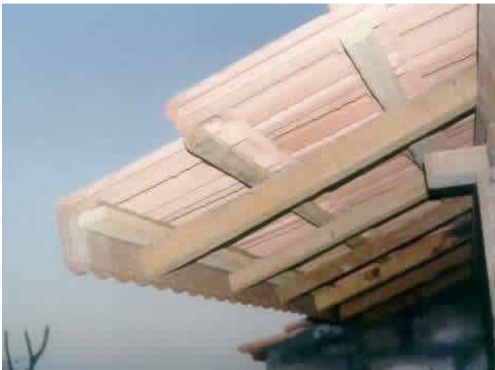
Critical Structural Details: Mangalore Tile Roof Construction (Source: Sudhir K. Jain, IIT Kanpur)
