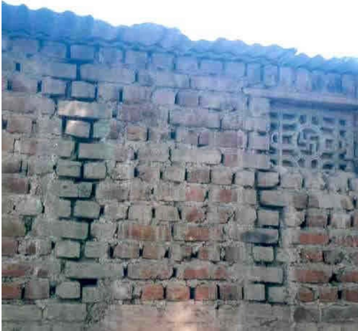
Critical Structural Details: Elevation of Brick Masonry Wall in Mud Mortar (Source: Svetlana Brzev)
