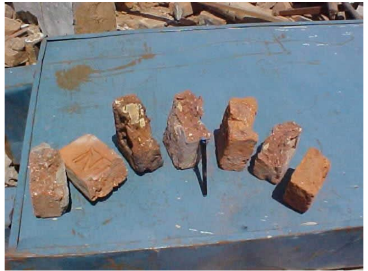
Construction Deficiency: Poor Quality Bricks (Source: Sudhir K. Jain, IIT Kanpur)
