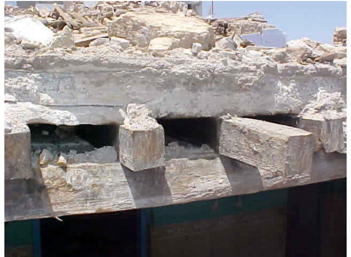
Key Seismic Deficiencies - Heavy Roof
