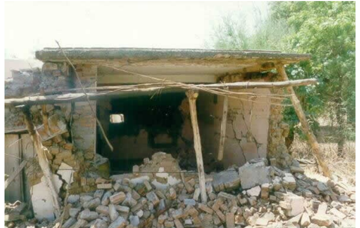
Typical Earthquake Damage - Failure of Masonry Walls in the 1997 Jabalpur Earthquake (Source: Sudhir K. Jain, IIT Kanpur)
