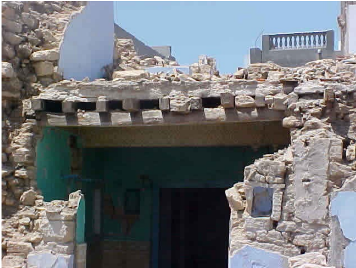
Typical Earthquake Damage in the 2001 Bhuj Earthquake (Source: Sudhir K. Jain, IIT Kanpur)
