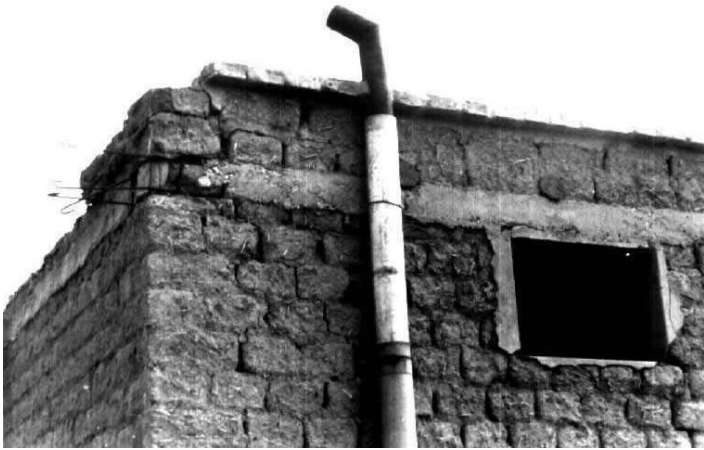
Photograph illustrating typical earthquake damage
