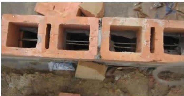
Horizontal reinforcement placed in between the horizontal bed joints. (2 bars of 4mm diameter) (August 2011) [1].
