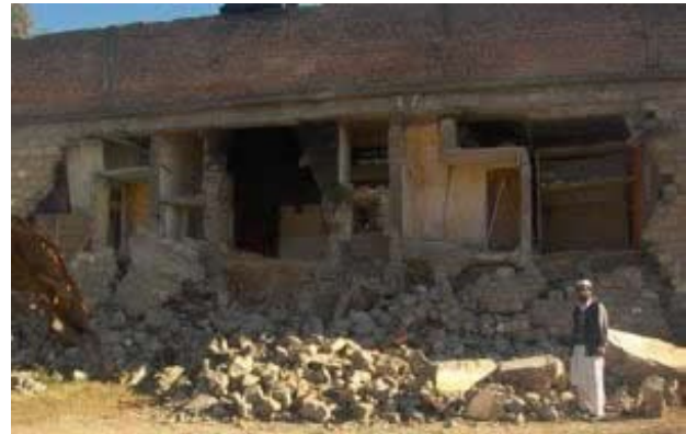
Out of plane flexural failure of load bearing wall constructed with block masonry in Kashmir Earthquake of 2005 [4].
