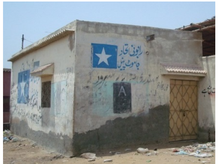
Block masonry with CGI sheet roof held down by a plastered parapet of blocks.
