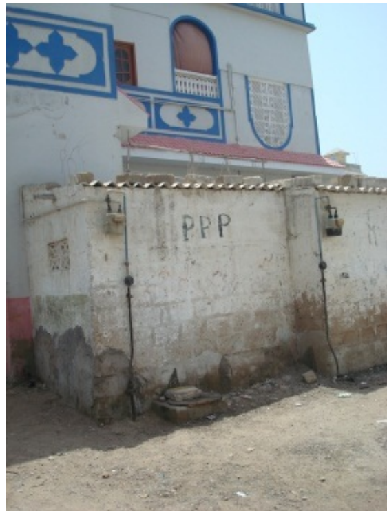
Adhoc appendage to the building.
