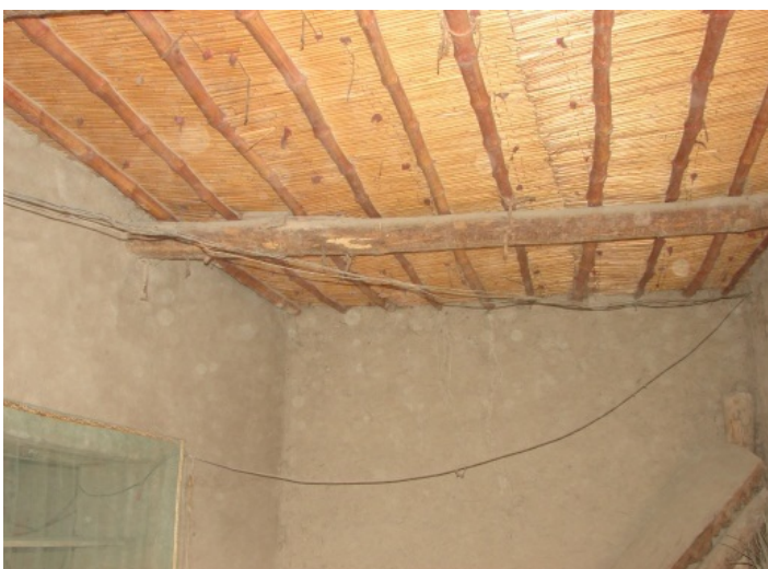
Adobe house roof - interior. Timber planks with bamboo stalks supporting wooden chick.
