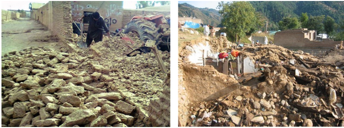
Typical damage caused by the Dalbandin earthquake in 2011.
