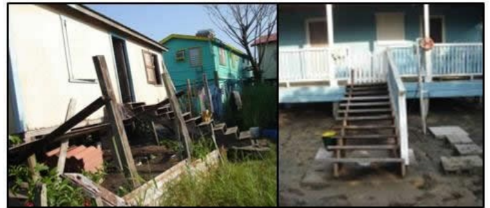
Stilt houses fell off their timber posts during the 2009 earthquake
