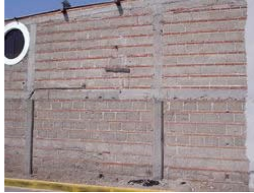
Combined and confined masonry house: 1 course of bricks alternate with 1 course of concrete blocks.
