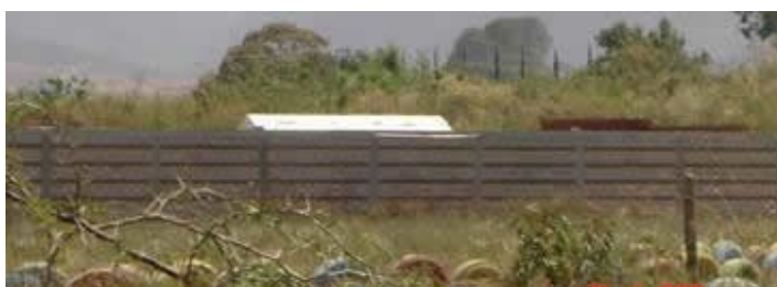
Combined and confined masonry fence: 2 courses of bricks alternate with 3 courses of concrete blocks.
