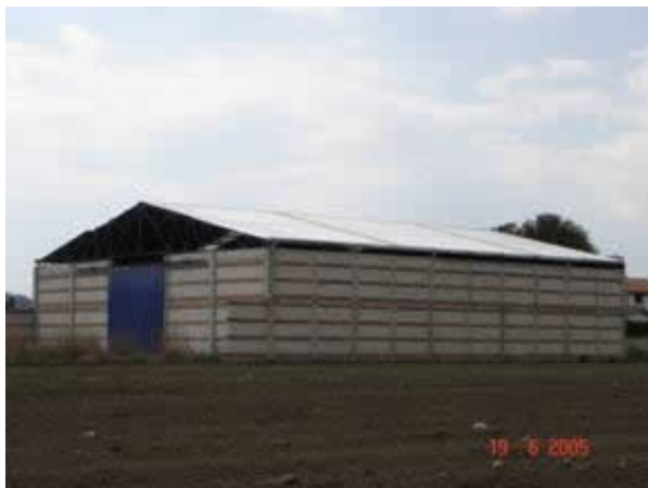
Combined and confined masonry warehouse: 3 courses of bricks alternate with 3 courses of concrete blocks.
