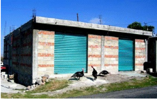
Combined and confined masonry store: 2 courses of bricks alternate with 2 courses of concrete blocks.
