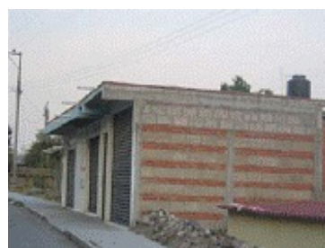
Combined and confined masonry store: 2 courses of bricks alternate with 1 course of concrete blocks.
