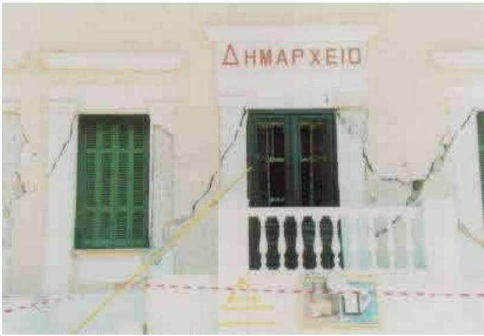
Typical Earthquake Damage - Shear Cracking of Masonry Walls (1999 Athens earthquake)
