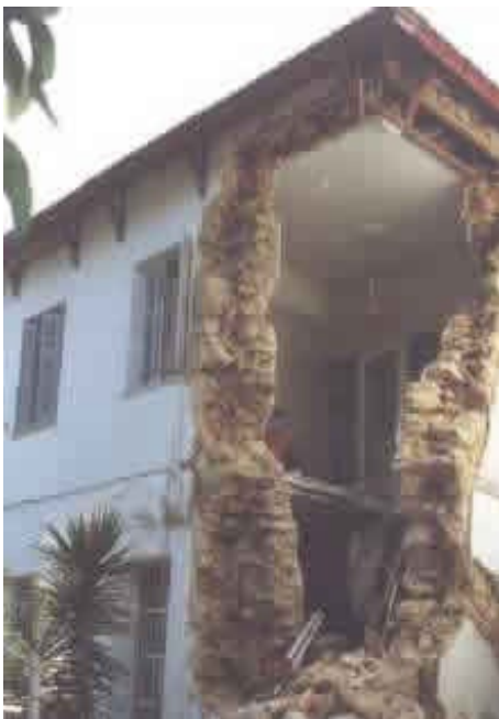
Partial Collapse of a Stone Masonry House in Nea Philadelphia (1999 Athens earthquake); Source: EERI
