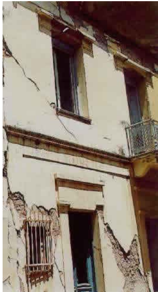
Typical Earthquake Damage - Falling of Plaster and Shear Cracking of the Walls (1999 Athens Earthquake)
