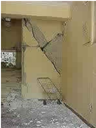
Failure of column, due to short column effect, of a 5-story building in Ano Liosia, which was built in 1997 according to the new Greek Seismic Code (1999 Athen earthquake); Source: ITSAK
