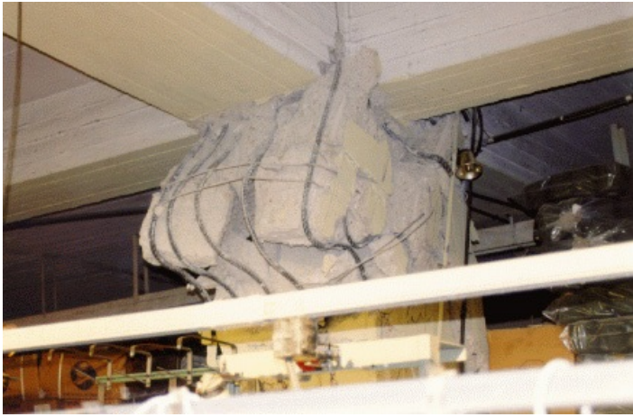
Earthquake Damage - Dislodged Column due to Soft Ground Floor Effect (1999 Athens earthquake)
