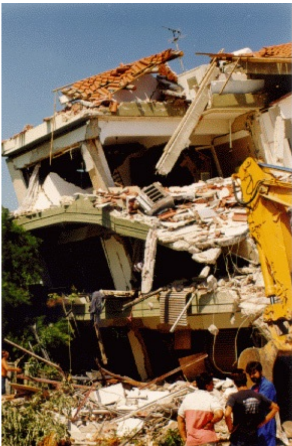
Typical Earthquake Damage (1999 Athens earthquake)
