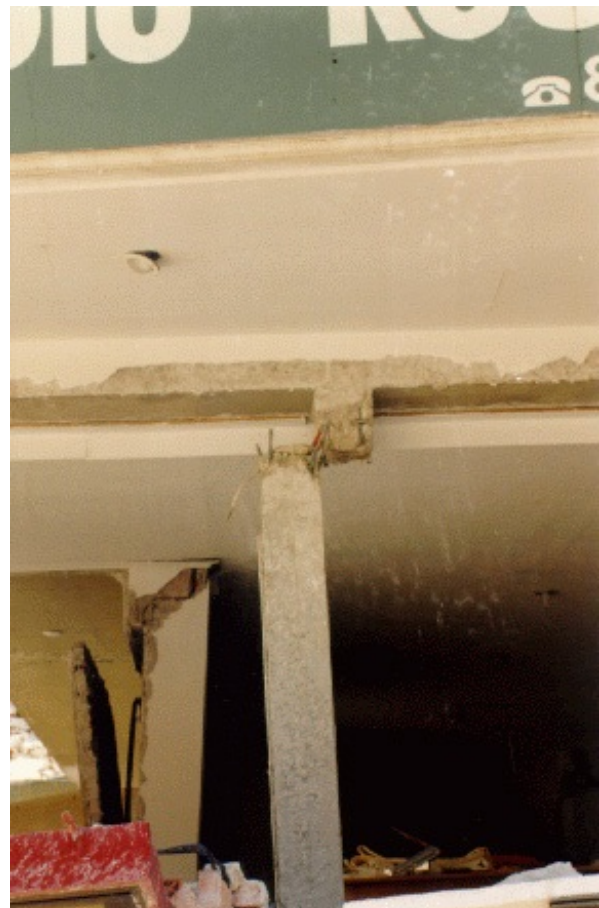
Building Collapse in the 1999 Athens earthquake
