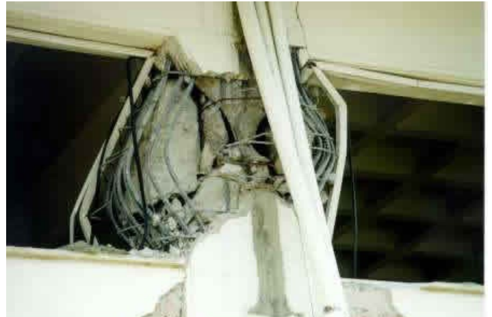
Typical Earthquake Damage-Column Failure (1999 Athens Earthquake)
