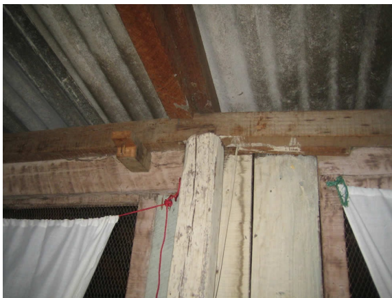
Roof made of asbestos sheets supported by wooden beams which loosely rest on the wooden walls.
