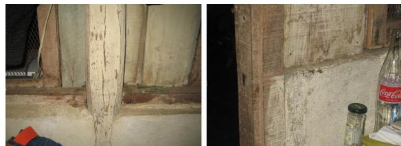
Detailing of the transition zone between the masonry base and upper wooden part of the wall.
