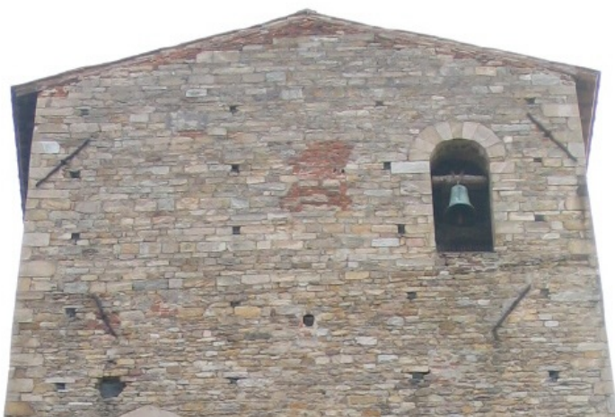
Opposite walls are connected by the use of tie-rods, with evident improvement in seismic behavior.
