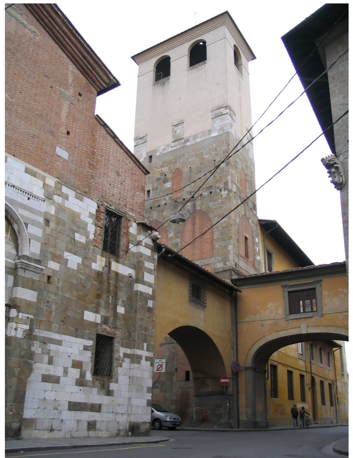
"Torre della Verga d'oro." Structural reinforcements: two large arched openings supporting horizontal forces at the base of the tower have been infilled by clay units.
