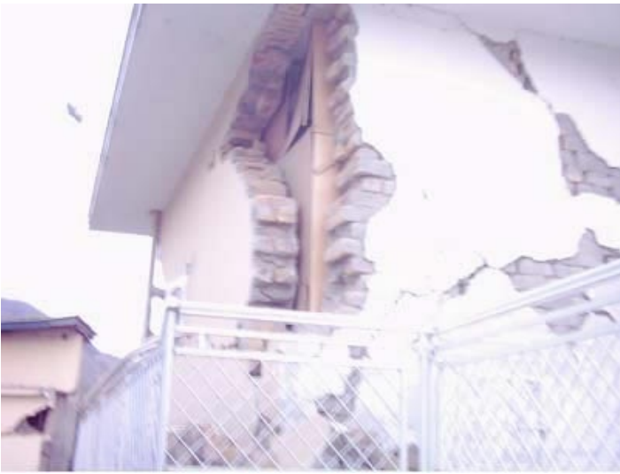
Corner failure in in a two story brick masonry house at Muzaffarabad, Kashmir, (from Kashmir earthquake Oct 08, 2005)
