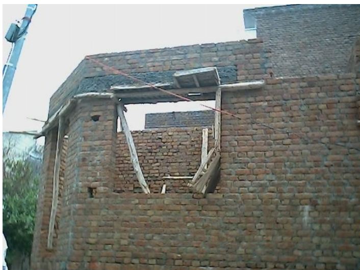
Discontinuity of lintel beams
