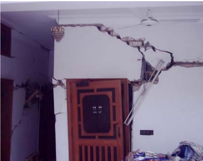
Cracks above door opening and along lintel in a 4.5 inch (125 mm) thick wall in a partition w all in a house at Muzaffarabad, Kashmir, (from Kashmir earthquake Oct 08, 2005)
