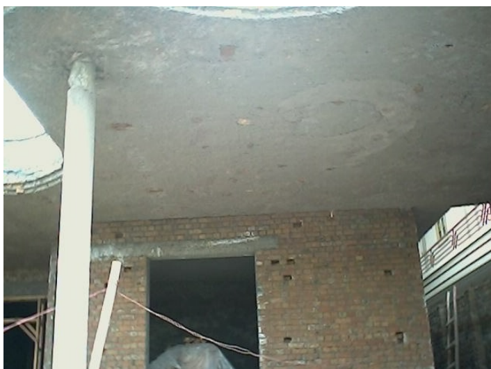
Poor quality of RC work in roof slab (A large number of bricks are placed in RC work to save cement concrete)
