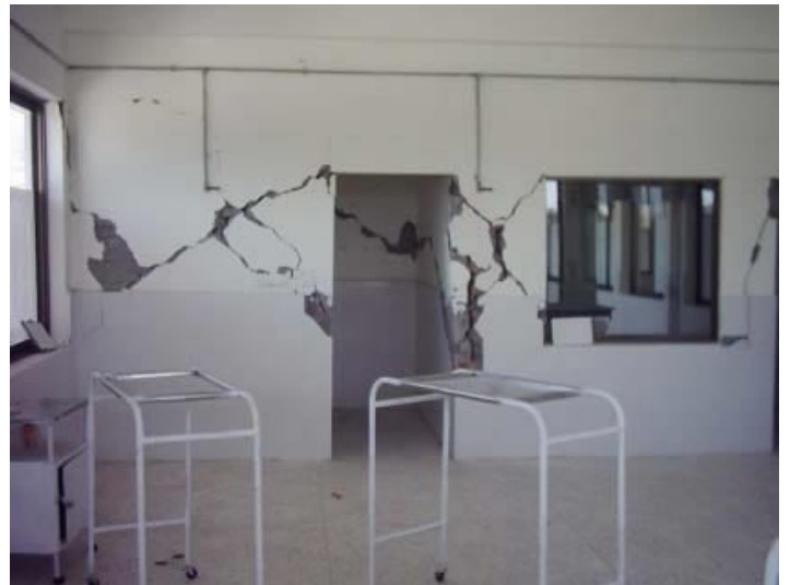
Typical cracks in pier: Manserhra Hospital NWFP Pakistan (from Kashmir earthquake Oct 08, 2005)
