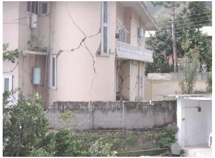
Typical Scissor type cracks in a two story brick masonry house at Muzaffarabad, Kashmir (from Kashmir earthquake Oct 08, 2005)
